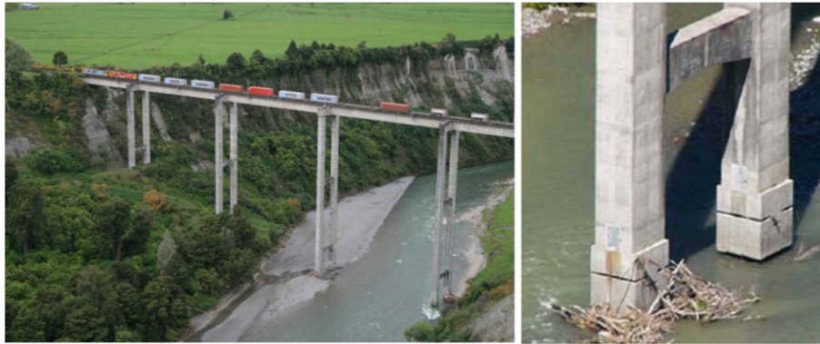
FIGURE 2 View of the South Rangitikei Rail Bridge in New Zealand. The piers are allowed to uplift by 12.5 cm; while the rocking motion is controlled by torsionally yielding steel-beam dampers shown in Figure 3 [Colour figure can be viewed at wileyonlinelibrary.com ]
